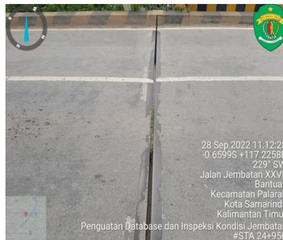
Gambar 5. Expansion joint abutmen terisi pasir
